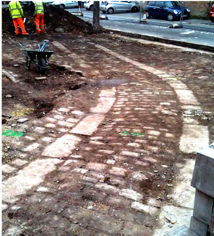
Plate 6.1 Road surface as excavated
